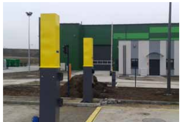
PI-MSKA system with two detectors placed opposite each other
